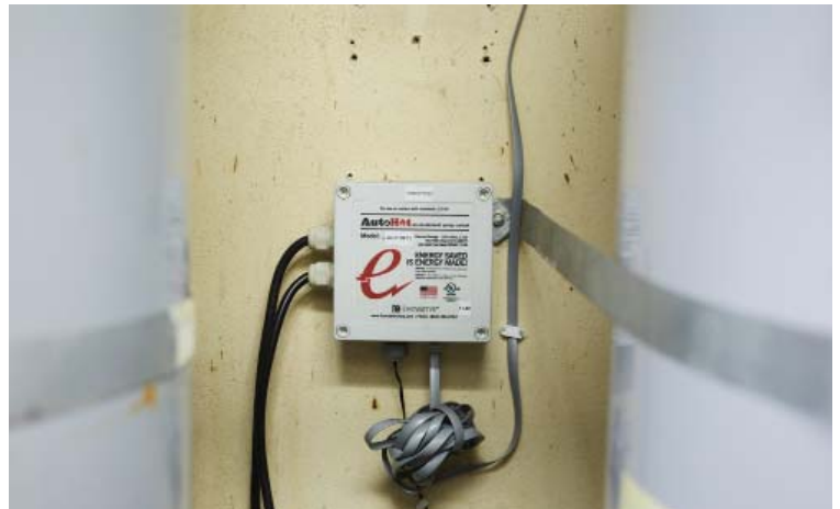
Hot water recirculation controls supplies hot water quickly, reducing wasted water
